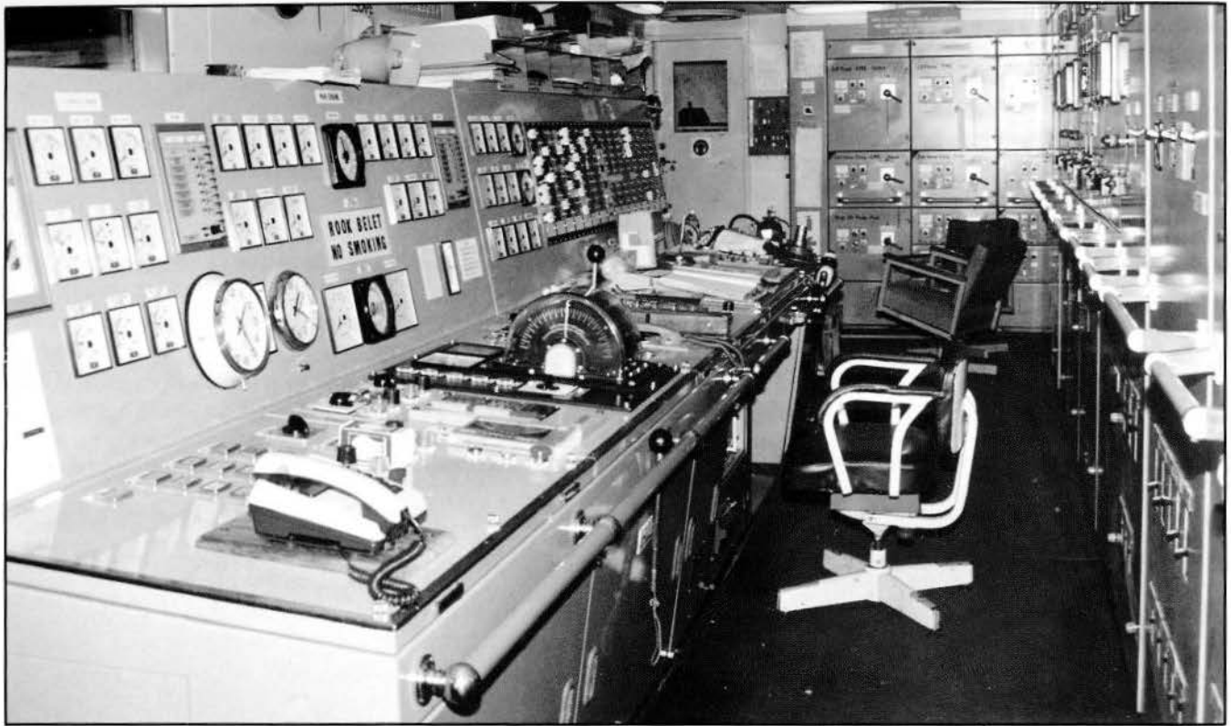
Fig 2 The engine room of the SA Agulhas
