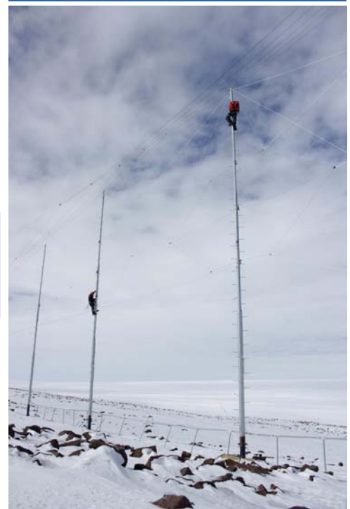
The new Antenna array of the HF Radar at SANAE-IV. The Twin folded dipole array replaced the previous 16 element Log-periodic array which was demolished by strong winds in 2008.
