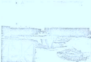
"Main Street" of Little America V under construction on the Ross Ice Shelf during the 1955-1956 season.
