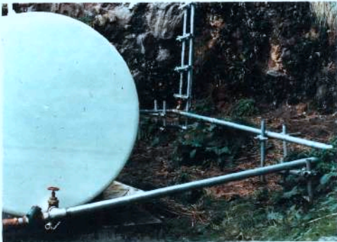
A NEW BY-PASS DIESEL LINE WAS INSTALLED FROM THE LOWER DIESEL TANK AND PUMPHOUSE TO THE TOP OF THE CLIFF WHERE IT WAS JOINT TO THE EXISTING LINE
