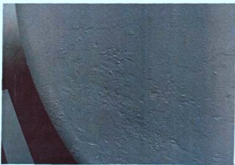
VIEW OF PITTING WHICH IS TAKING PLACE ON THE SHELL OF THE FOUR (4) FURTHERMOST DIESEL BULK STORAGE TANKS
