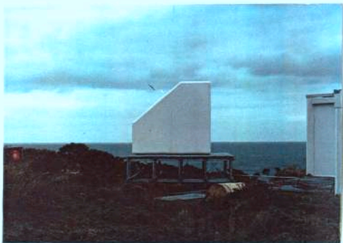
VIEW OF THE PIPE FOUNDATION AND THE COMPLETED SATELLITE BUILDING WHICH IS SITUATED NEXT TO THE BALLOON HUT.
