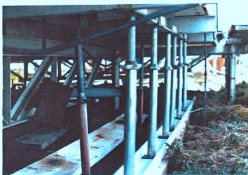
FLOOR OF THE HYDROGEN GENERATOR ROOM WHICH WAS IN THE PROCESS OF COLLAPSING. THIS HAS BEEN RECTIFIED WITH STEEL BRACING.
