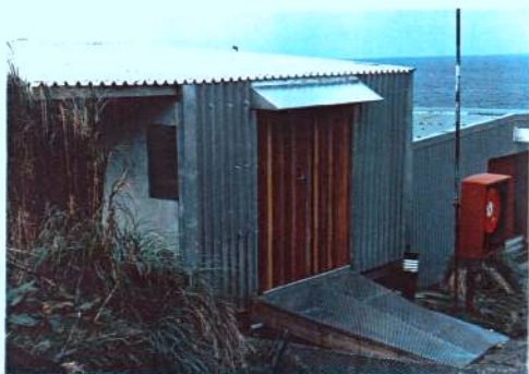
VIEW OF THE POWER HOUSE WHERE THE WINDOW WAS REMOVED AND NEW WOODEN DOUBLE DOORS WERE INSTALLED
