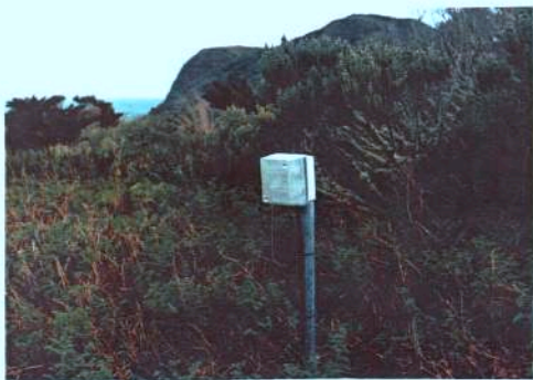
VIEW OF THE LOW DENSITY TYPE LIGHT FITTINGS INSTALLED BESIDE THE CAT-WALKS FROM THE HELIPAD TO THE PWD STORE
