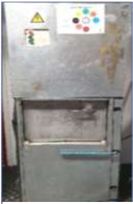
Figure 8: Waste Room compactor.
