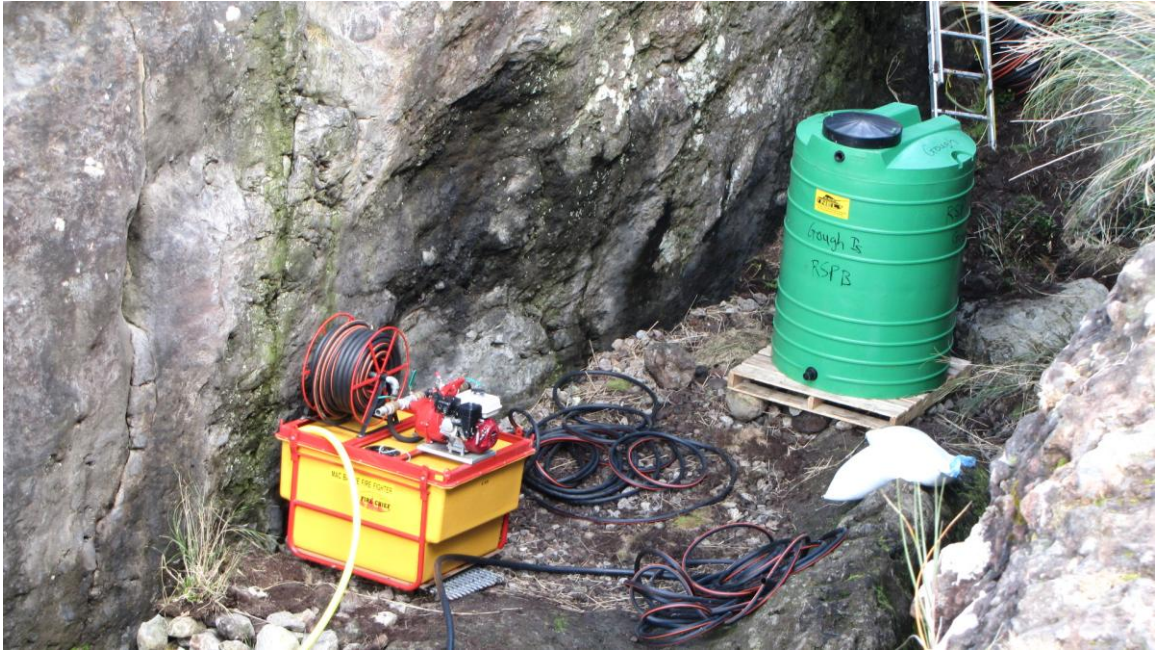
Fig. 5. Water pump and salt-water storage tank at Snoekgat
