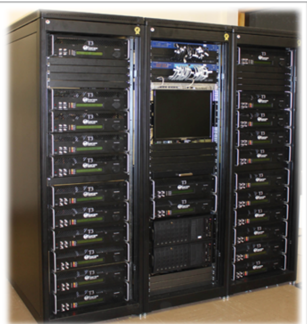
4. Each antenna is driven by a digital transceiver box, responsible for transmitting and receiving the signals controlled by a server.
