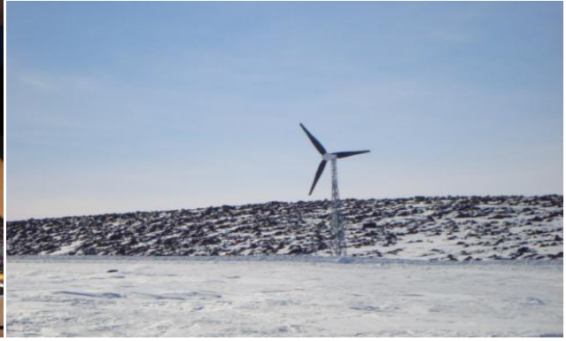
Figure 17: The wind turbine.
