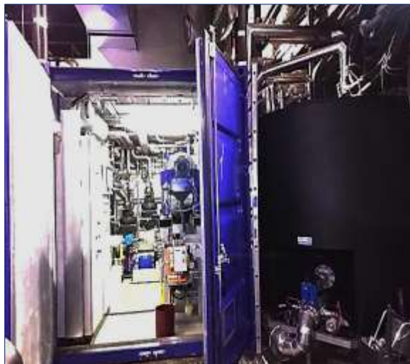
Figure 6. Inside of MBR plant plus sludge tank on the right.
