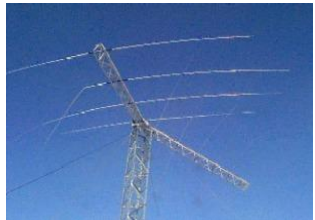
A wind damaged radar antenna.
